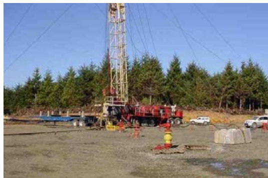
Exploration for methane in 2006 on Beaver Hill near Coquille. Four wells were drilled and tested.
