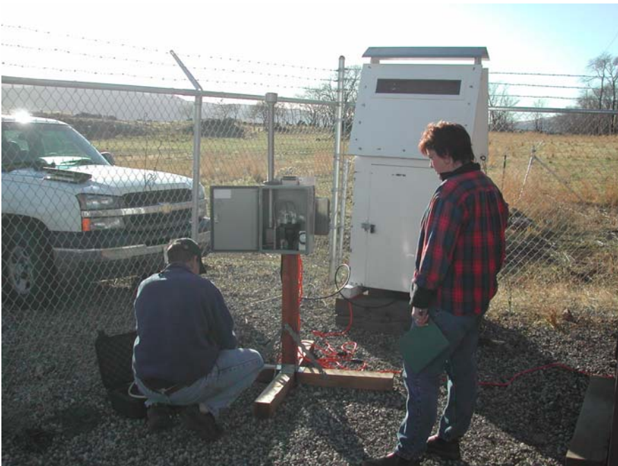
Installation of IAS sampler at Towal Road – Dr. Steve Cliff on left and Jackie Brown on right
