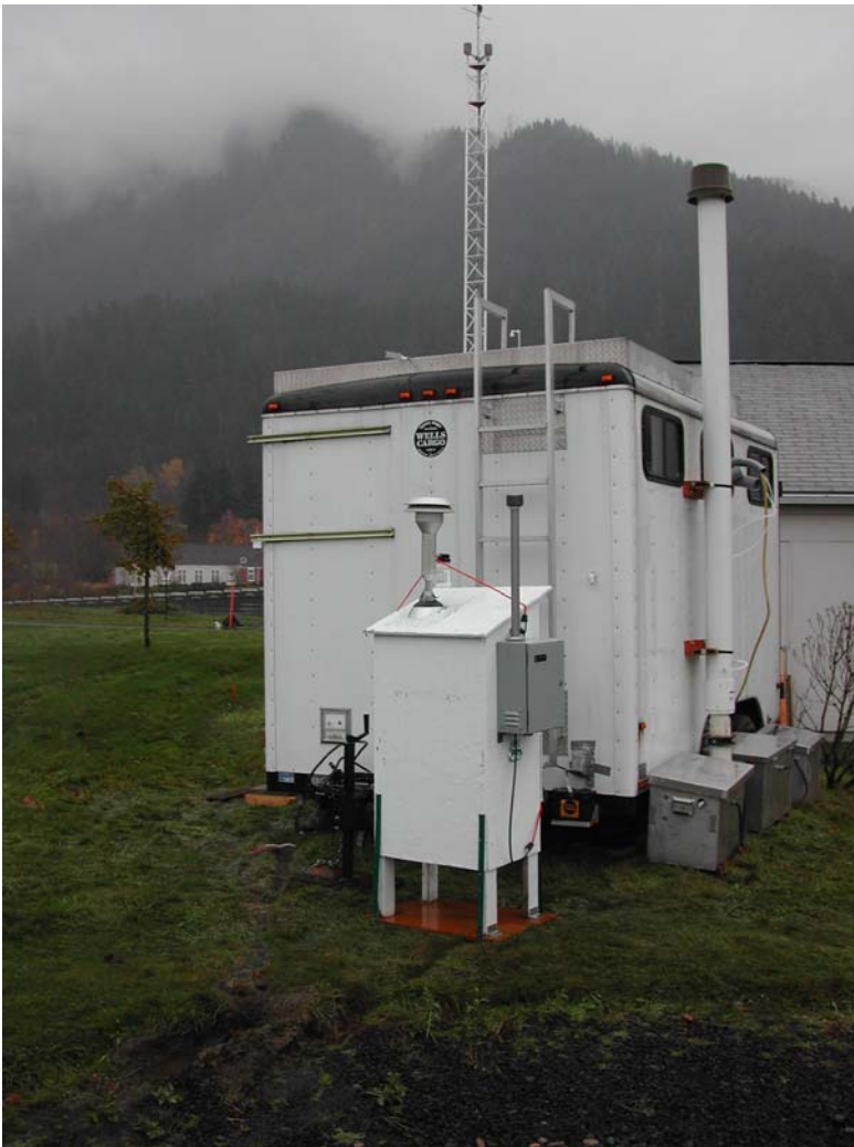
IAS/DRUM sampler in foreground with monitoring trailer at Bonneville Dam – meteorological station and nephelometer in building behind trailer.
