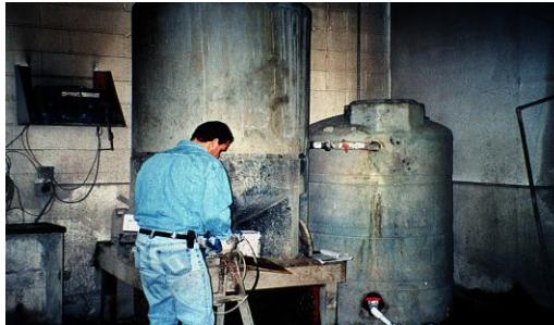
Mac's Radiator initiates the installation of their zero discharge wastewater treatment system.
